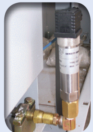
SF 6 Density Sensor Installed on Fill Port
